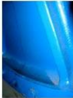
Photo 25: leakage Input shaft BS
