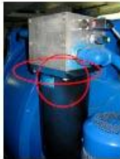
Photo 27: leakage oil filter manifold
