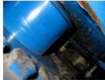
Photo 26: leakage high-speed shaft GS
