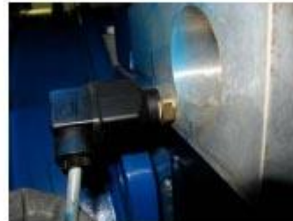
Photo 28: damage to pressure sensor (loose) on oil filter manifold
